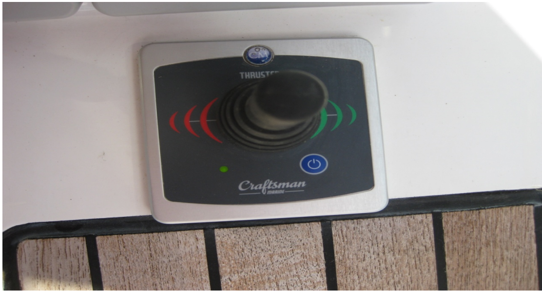
BOW THRUSTER CONTROL PANEL, ON COCKPIT AREA
