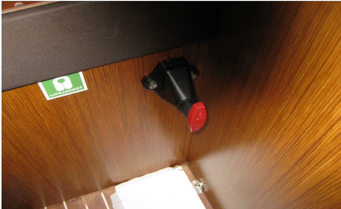
Bow-thruster switch is in ON position as is shown to the above photo Location: In the front port cabin
