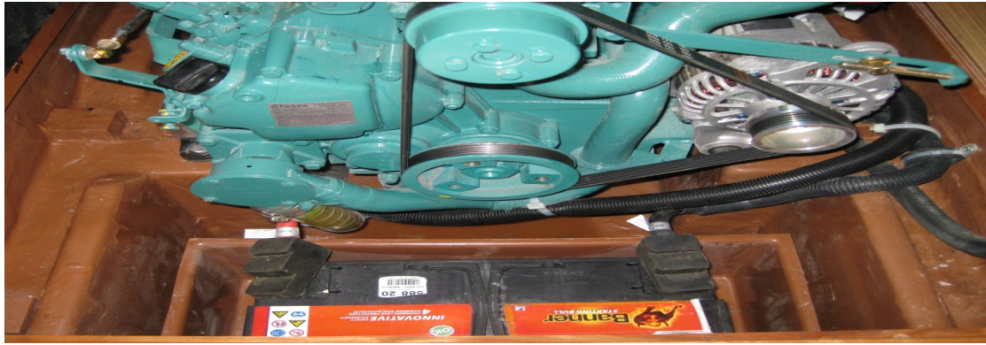
Starter battery is placed into the motor room V.H.F. Emergency Battery
